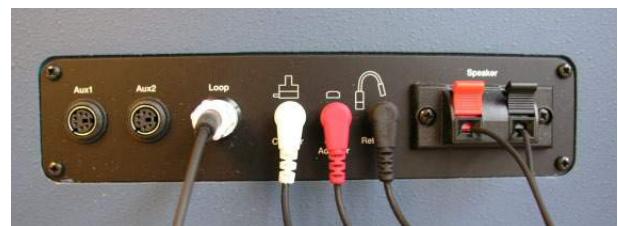
Figure 3: Cable placement in TBS25
